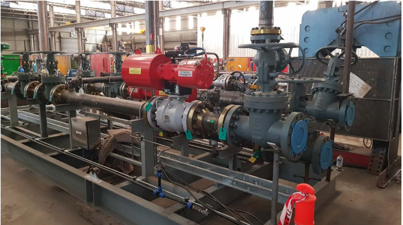
Modularised Syngas control valves
