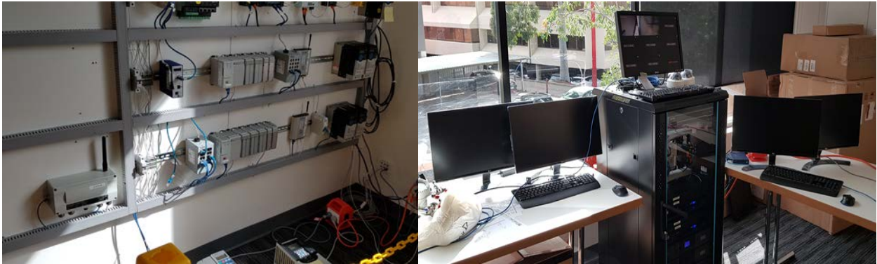
PLC Control System undergoing testing by ATSys
