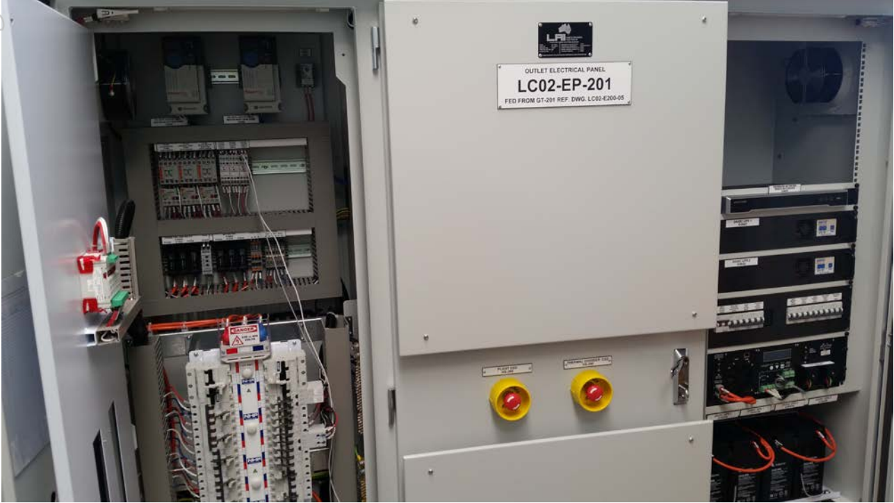
Electrical Panel undergoing Factory Acceptance Testing by ATSys
